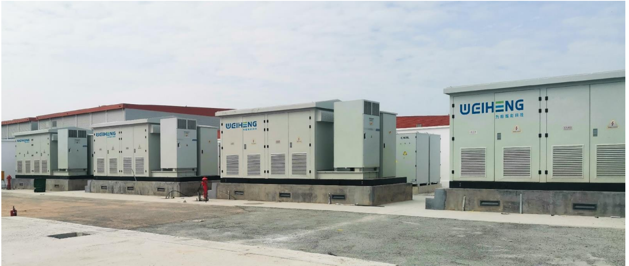
Reference case in Guangdong, China • GAC CATL Energy Storage Project – 12MWh
