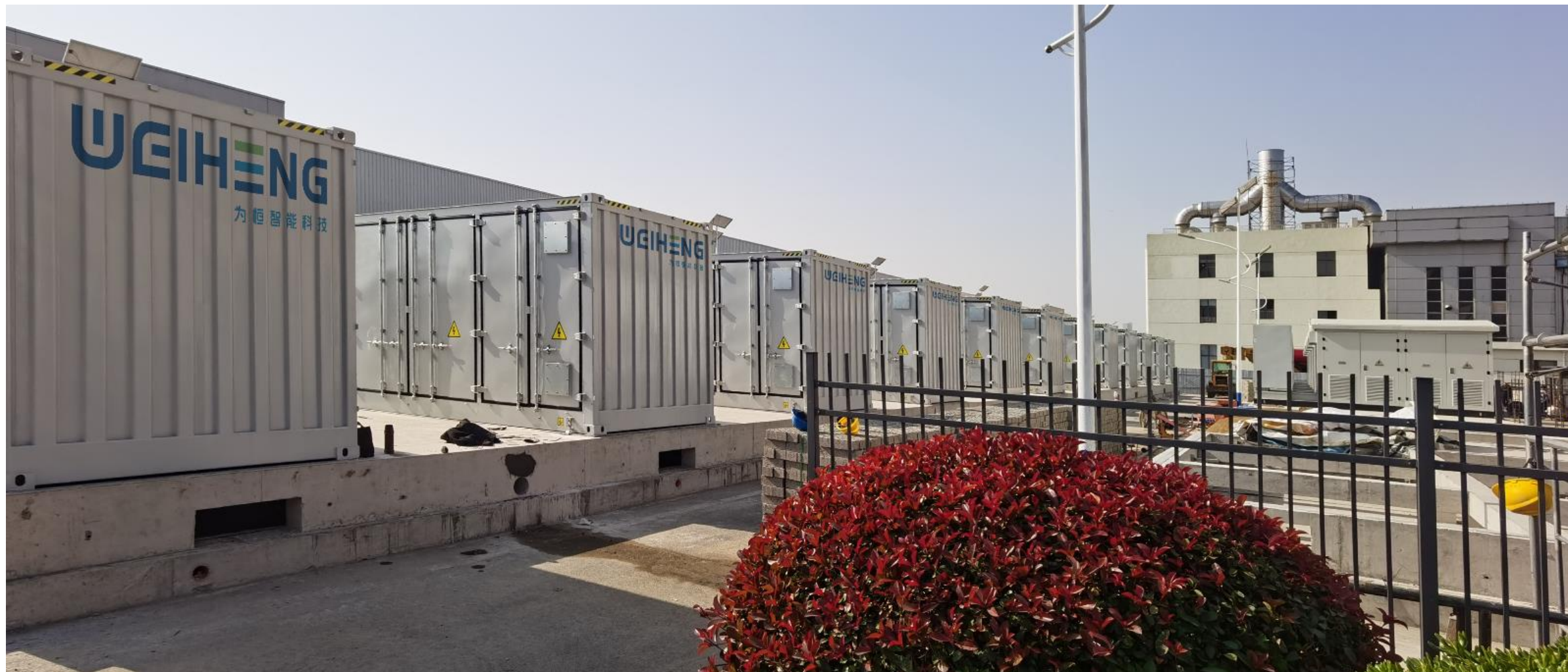
Reference case in Jiangsu, China • KEENSTAR Energy Storage Project - 40MWh
